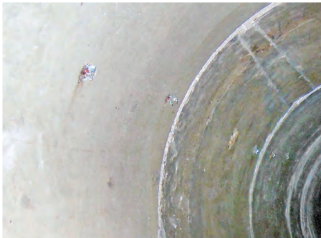
Cable clips inside the tunnel
